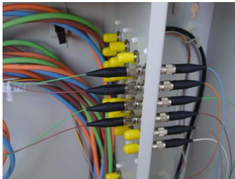
Fiber Optic Cable Terminations
